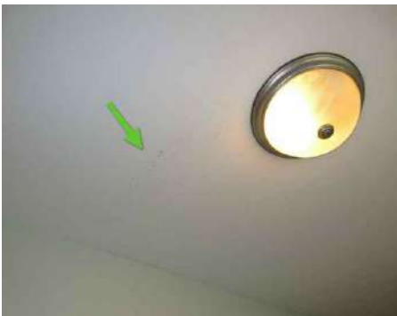
Peeling paint - ceiling (near exterior basement entrance)
