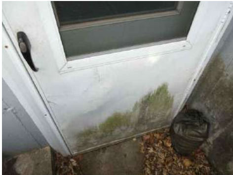
Corroded storm door - lower-level entrance
