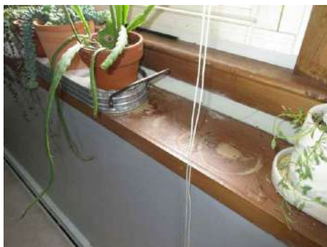
Moisture stains on windowsills appear to be from water plants - consult owner to confirm
