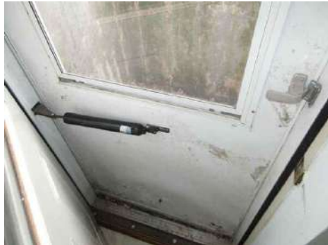
Corroded storm door - lower-level entrance
