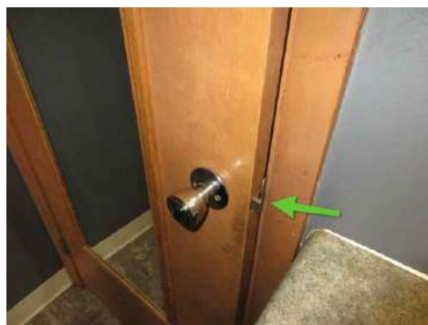
Bath door does not latch/lock
