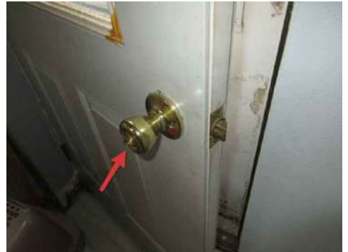
Door does not lock - lower level door
