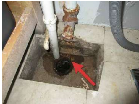
Open drain for laundry sink and washer drain - not recommended
