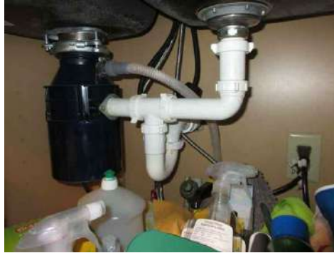
Kitchen - recommend disposal have its own trap
